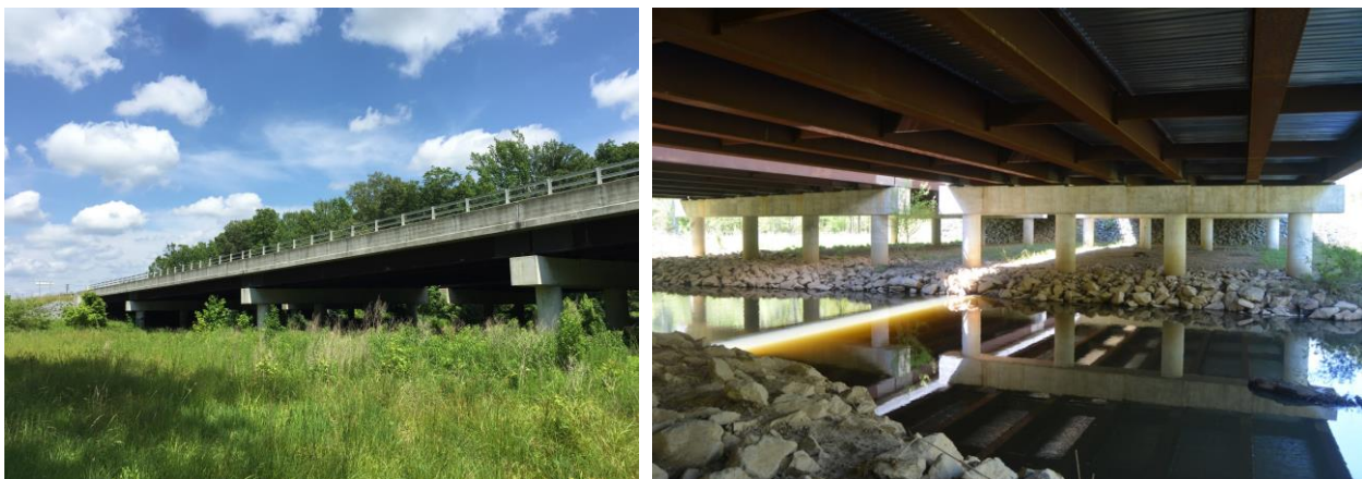
Figure 2. Bridge lengthening over New Hope Creek on 15-501 in Durham, NC. This underpass was extended on either side of the river to improve wildlife movement through this important habitat corridor.
