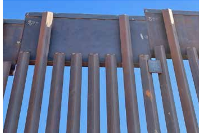
Note each panel consists of 8 six-inch steel bollards with four inch spaces between each bollard.
