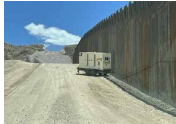
Construction equipment left unsecured. Generator had slid down the slope and lodged in fence. May 21, 2021. 31.445811, -111.427886. Photo: Myles Traphagen
