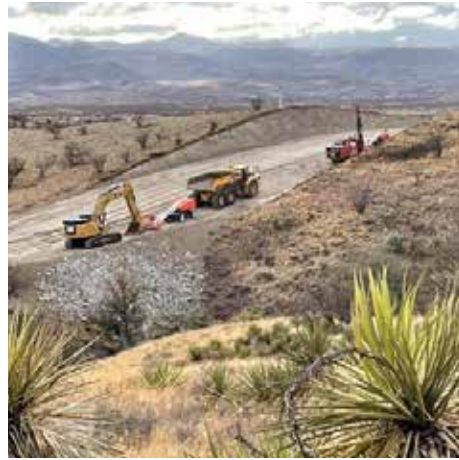
Looking west into Coronado National Forest at Roosevelt Easement border wall site. Note filled in drainage. Jan. 21, 2021. 31.333623, -110.782415
