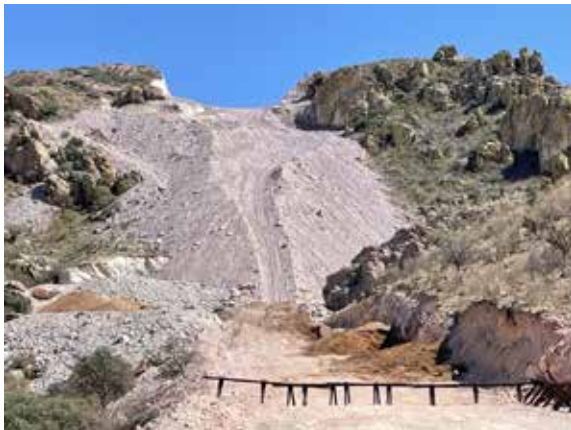
Looking east into Coronado National Forest at Cerro del Fresnal border wall site. May 25, 2021. 31.333623, -110.782415. Photo: Myles Traphagen
