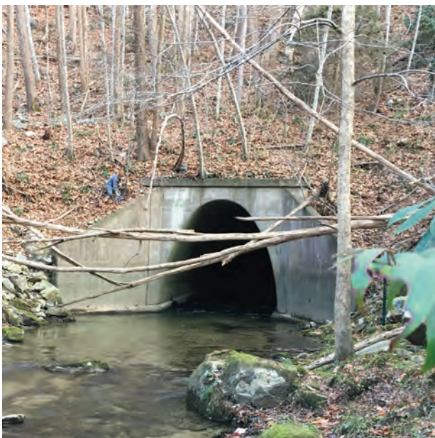
Hurricane Creek Culvert. Photo: NPCA
