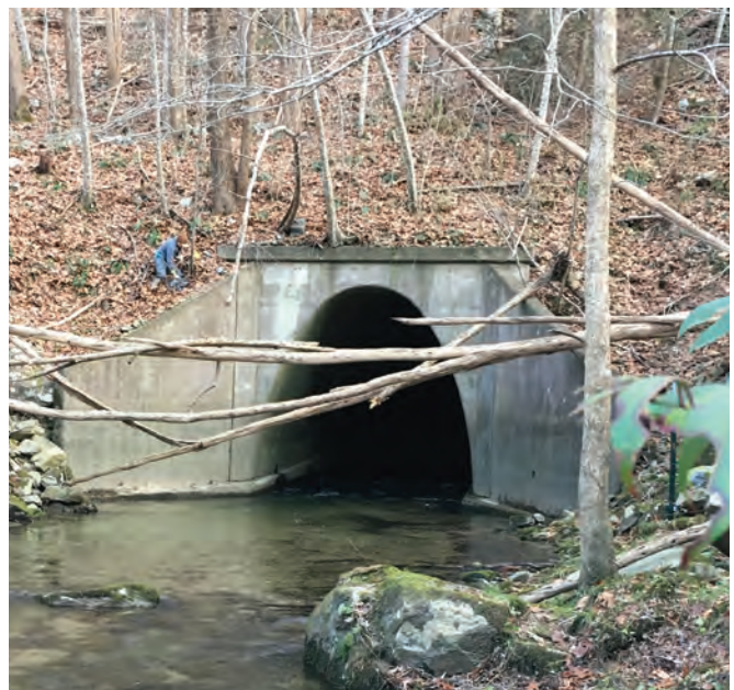
Hurricane Creek Culvert. Photo: NPCA
