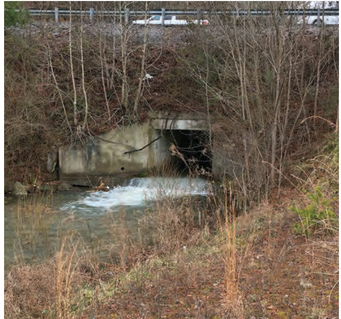
Millcreek A Box Culvert. Photo: NPCA
